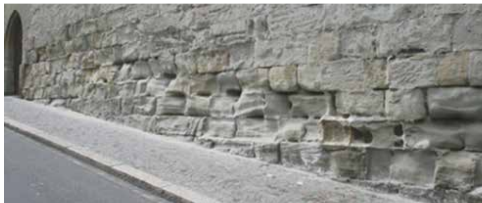
Figure 3: Lausanne (canton de Vaud, CH), rue de la Barre, Château Saint-Maire (10.04.2012). The sanding and disaggregation that affects the base of the building and up to 2 m in some areas is mainly due to the presence of NaCl.
