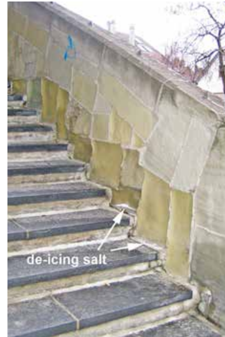
Figure 1: Lausanne (canton de Vaud, CH), Pierre Viret stairs (20.01.2010). Deicing salts are spread lavishly on the practically non-porous gneiss, and the salt and melted snow mixture accumulates at the base of the porous molasse-sandstone bridge wall that promptly powders and disaggregates.
