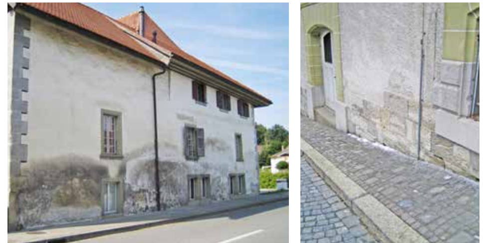
Figure 2: Left: Belfaux (canton de Fribourg, CH), north façade of the Lanthen-Heid manor (1526). The damages that affect the render and the underlying molasse-sandstone are mainly the result of splashing traffic along this street (3.09.2008). Right: Lausanne (canton de Vaud, CH), rue Saint-Etienne (20.01.2010). During dry winter cycles the residues of recrystallized deicing salts can be seen at the foot of façades that can either be mobilized and suspended in the air or enter the material when dissolved in water via hygroscopicity, rain, or more snow.
